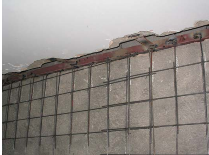
Figure 10. A typical view of the intersection between enhanced bearing walls and floor slab.
