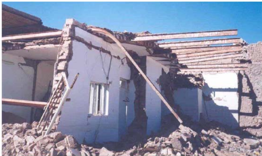
Figure 2. Damage to a traditional jack arch slab during Bam earthquake, 2003 [4].
