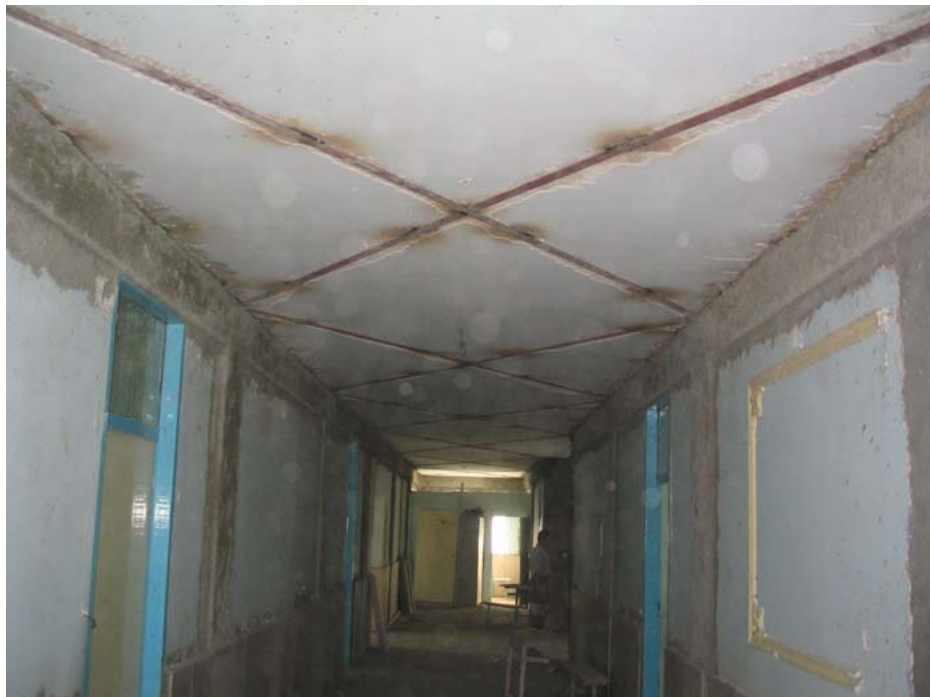
Figure 4. Adding 50 \times 5\text{mm} steel plates in order to integrate the traditional jack arch slab joists.
